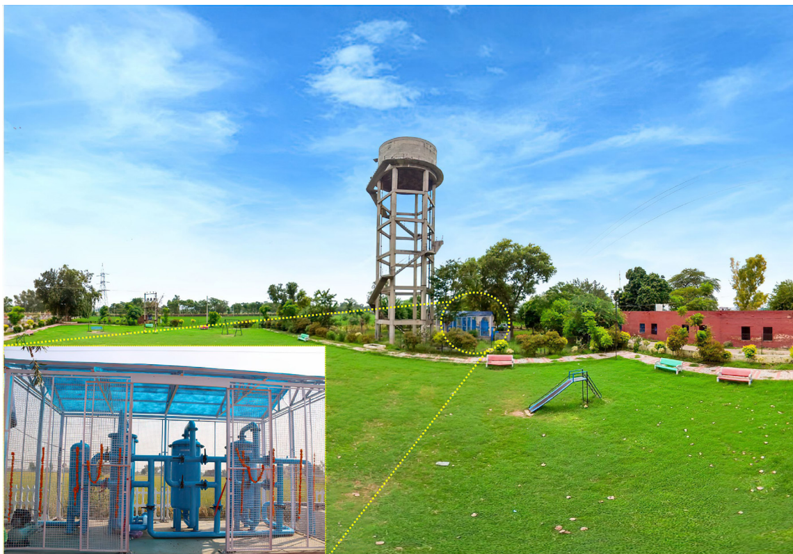
Figure 3. Photograph of AMRIT community unit installed in the state of Punjab, India. Oxidizer vessel through which air is pumped into the water for oxidation of Fe(II) to Fe(III), (B) Iron removal vessel for removing colloidal iron, (C) Arsenic removal vessel for removing arsenic (III and V) and (D) Polisher vessel for removing any foul smell or other impurities from the purified water. Microbial disinfection is also implemented if needed. The units are also monitored online with sensors for water quality and quantity. Implementations have been done by Hydromaterials Pvt. Ltd. (Detailed implementation of community units implemented in India can be accessed through the link: https://pradeepresearch.org/towards-an-arsenic-free-punjab-2/ )
